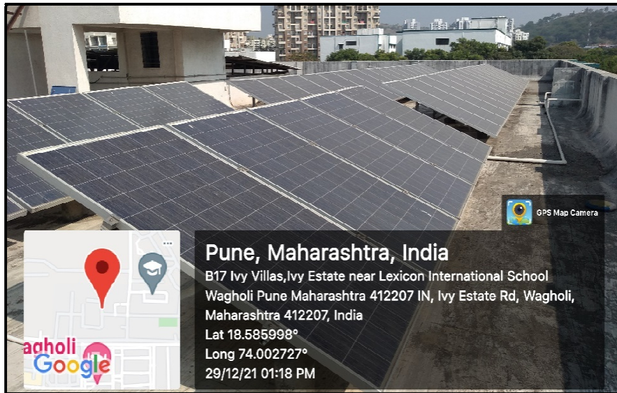
Photograph of Roof Top Solar PV Plant:
